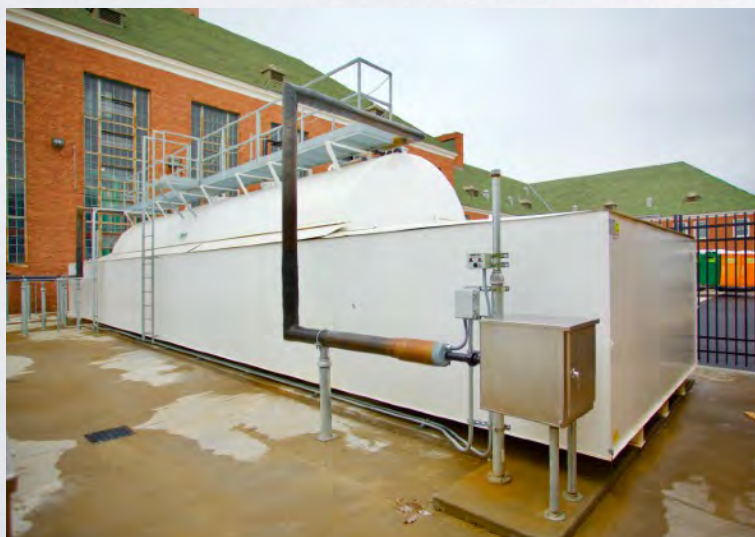
Highland Tank Secondary Containment
