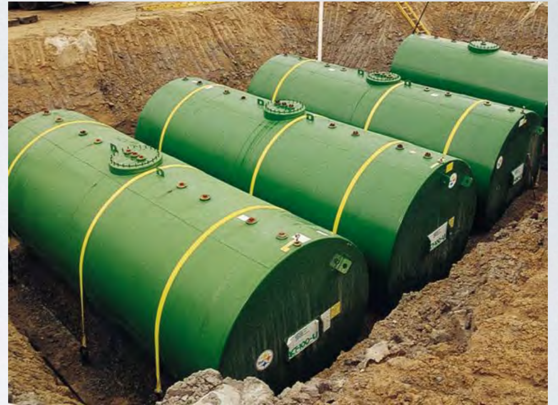
Highland Steel UST
